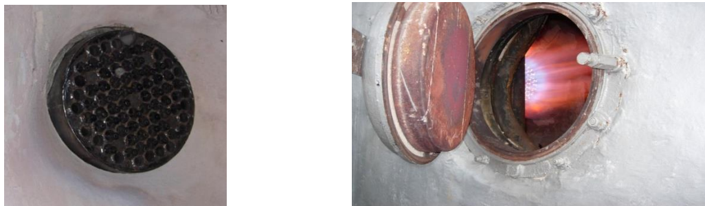
Figure 2 – View of the MIT burner in a boiler with a capacity of 10 MW and the nature of its flame
